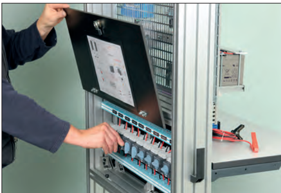
Flap for access to the switches
